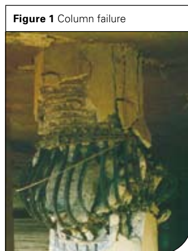
Photo courtesy of the New Zealand Society for Earthquake Engineering Reconnaissance Team Northridge 1994
